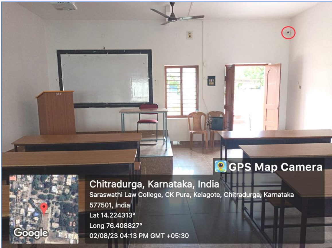
C.C Camera installed for the 3 rd Year LL.B Classroom surveillance
