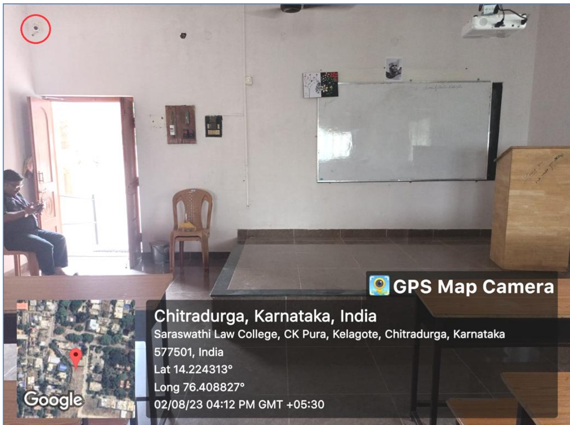
C.C Camera installed for the 1 st Year LL.B Classroom surveillance
