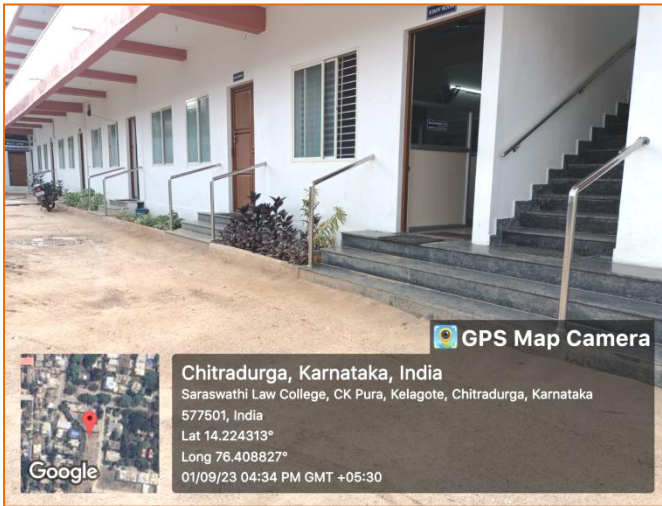
Railings are fixed to Administrative Off., Staff Room & Others to enter easily
