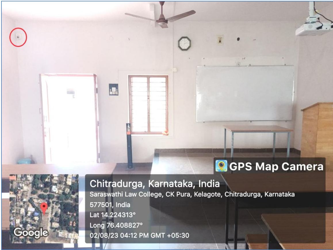
C.C Camera installed for the 2 nd Year LL.B Classroom surveillance
