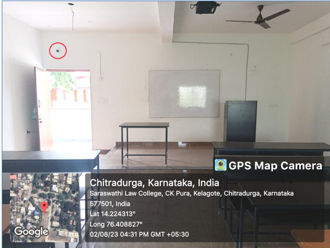
C.C Camera installed for the 2 nd Year B.A LL.B Classroom surveillance
