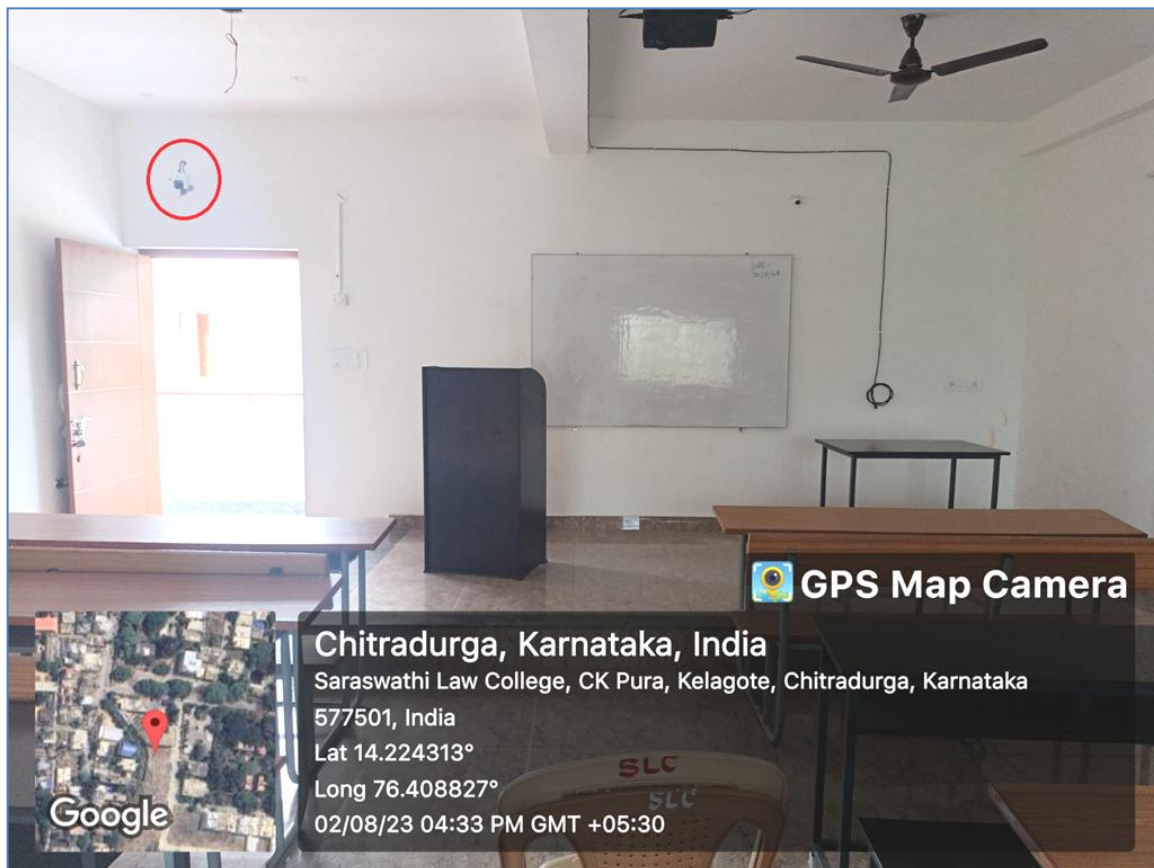
C.C Camera installed for the 3 rd Year B.A LL.B Classroom surveillance
