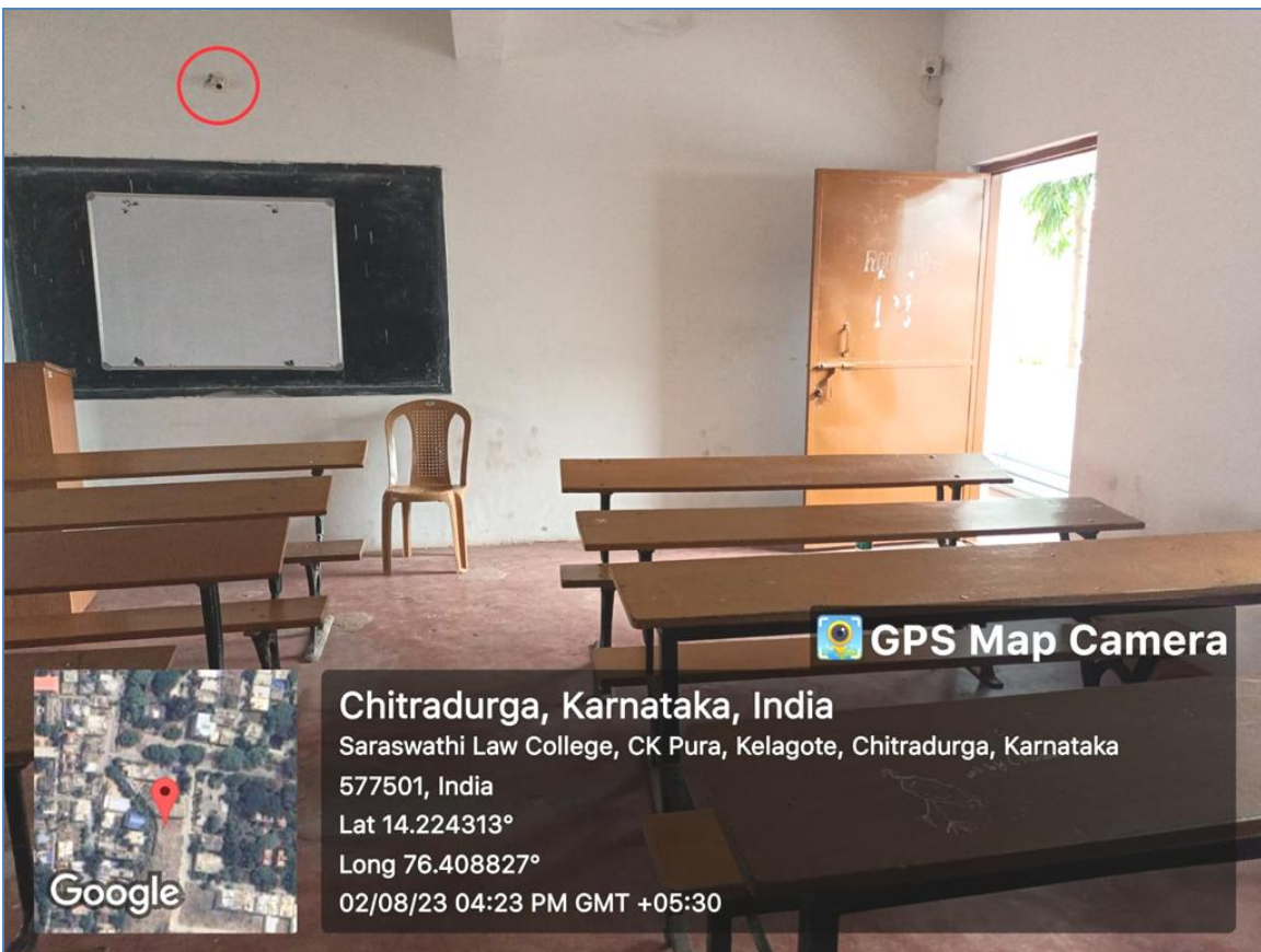
C.C Camera installed for the 5 th Year B.A LL.B Classroom surveillance
