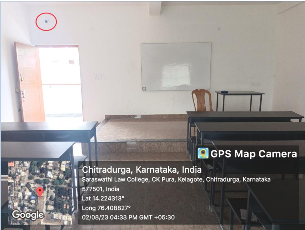
C.C Camera installed for the 4 th Year B.A LL.B Classroom surveillance
