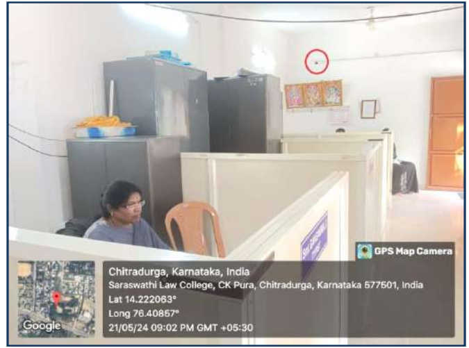
C.C Camera installed for the surveillance of Administrative Section of the Institution
