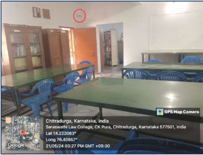
C.C Camera installed for the surveillance of Reading Room in the 2 nd entrance of Library
