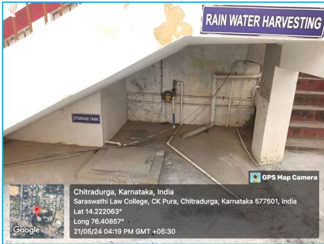
Rain Water Harvesting system
