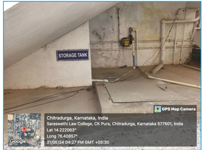
Water Tank to accumulate Rain Water
